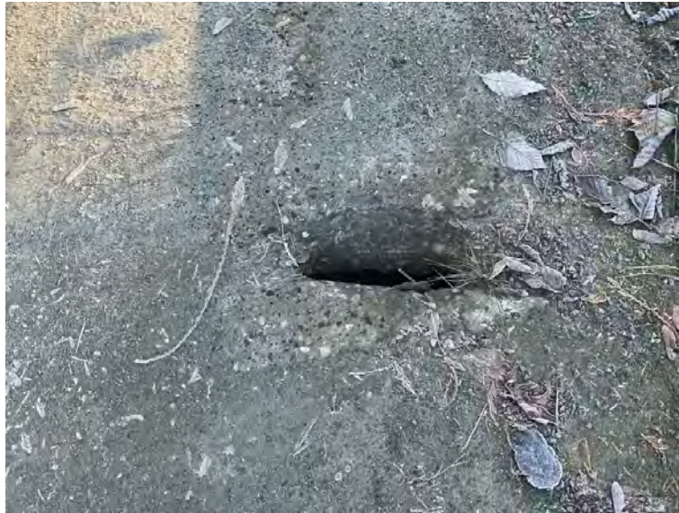
Downstream right bank concrete damage
