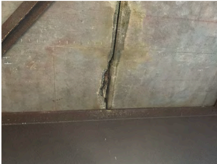
Upstream panel 1 right bank concrete damage
