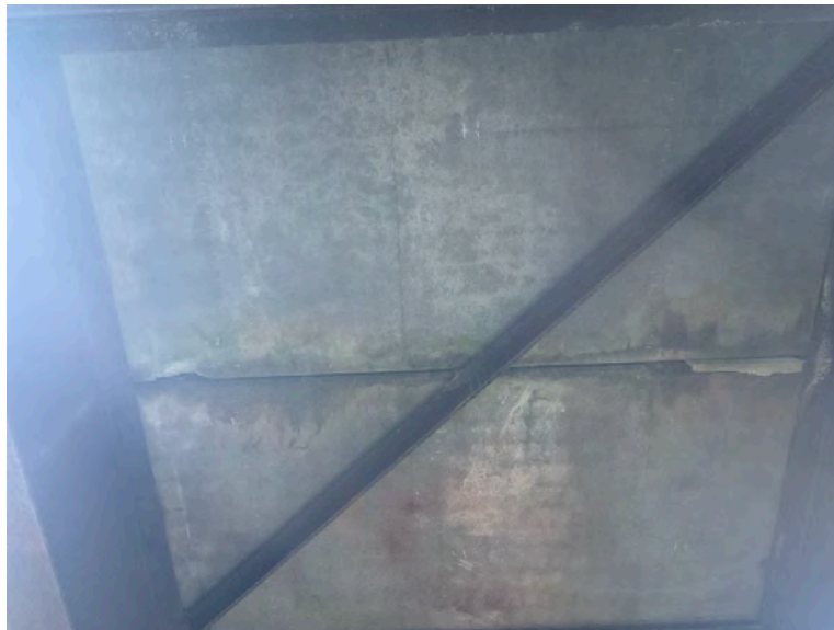
Concrete damage on panel 2 and 3
